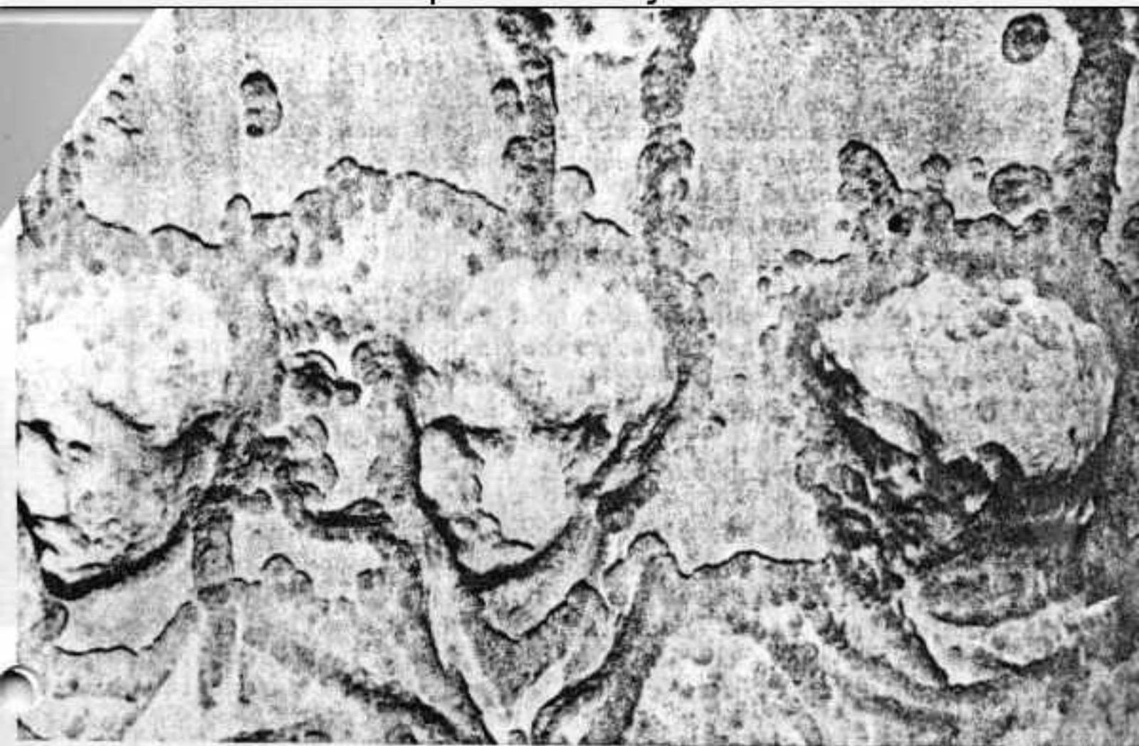
Fig. 1. Details of relief on Trajan's Column (in 1989) where the isolated pits are prominent on vertical parts and long depressions caused by joined pits or induced in a different way are common throughout.
